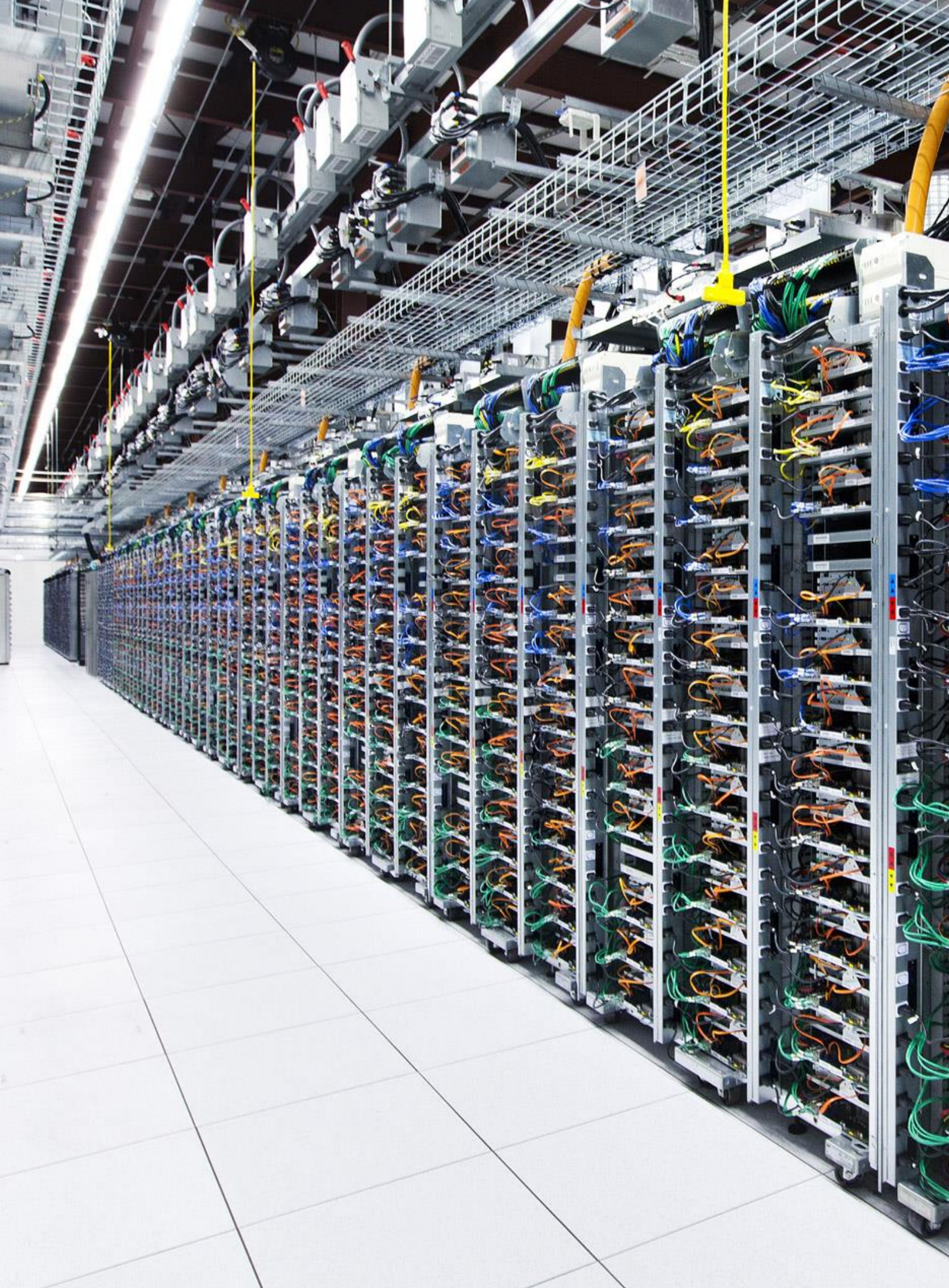
Inside a Google datacenter (Google, 2016)
